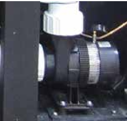
4) 24-hr Circulation Pump
